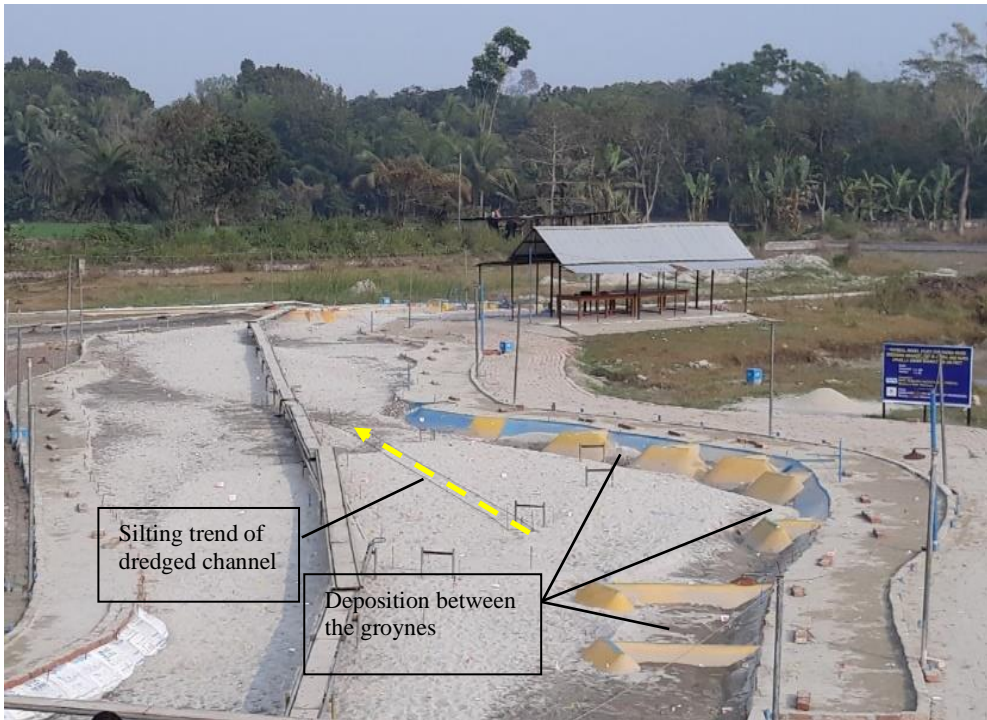
Fig. 5. Effectiveness of dredged channel, groynes & bank revetment as observed after model run (T6)
